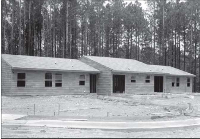
Left: Housing under construction for soldiers and their families. Over the years, many housing styles have evolved on Fort Polk.
