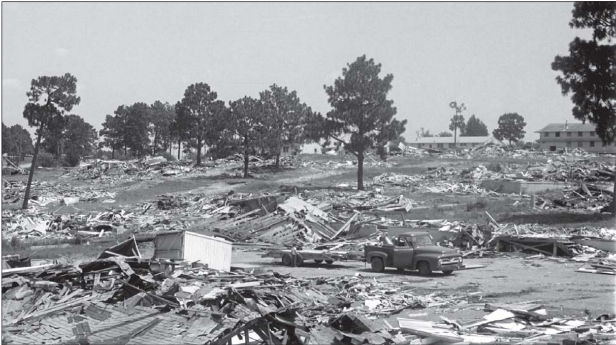
Below: In July 1976, building debris is cleared near Fort Polk's Youth Activity Center to make way for new construction.
