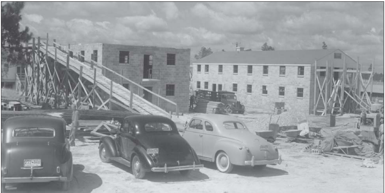
Below: Construction of Camp Polk took place at a feverish pace in 1941. Concrete block was used for some of the early buildings.
